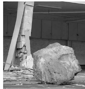
A boulder sits idle in a parking lot after it damaged support pillars of a Hawaii Kai town house.
